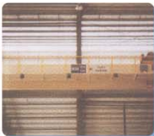
Hoist Crane(Double Girder)
