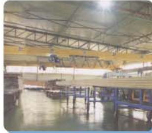
Hoist Crane(Single Girder)
